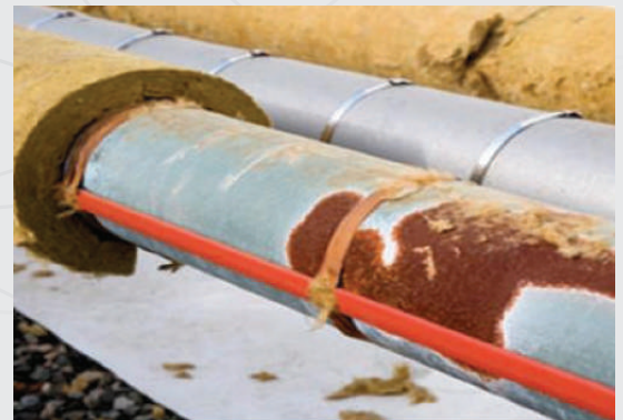
Localised CUI on coated pipeline
