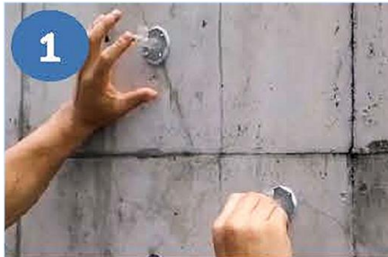
1 After measure the crack width, attach the packers with epoxy resin at approx. 200 mm spacing.
