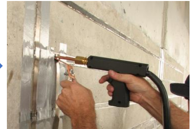
3. Connecting all MMO tape anodes to titanium conductor tape using spot welding.
