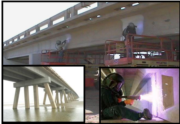
Figure 6. Thermally sprayed aluminum alloy galvanic anode installing on the prestressed beams and pile caps in Galveston, Texas.
