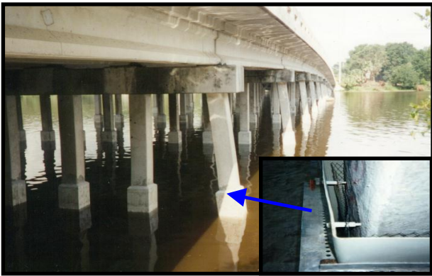
Figure 1. Pile jacket system installed on the prestressed concrete piles in Florida, USA.
