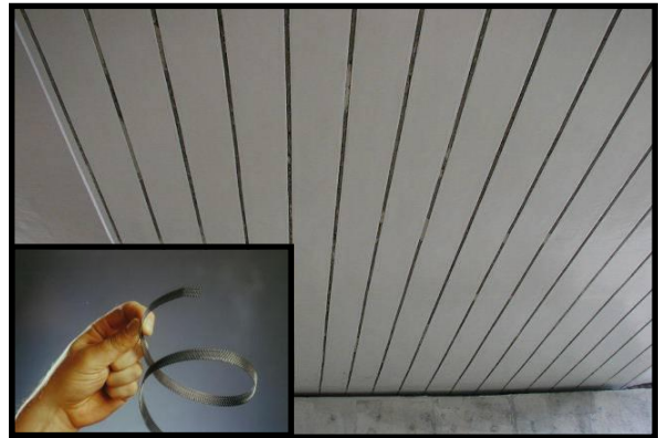
Figure 2. Titanium ribbon mesh anode slotted system installed on the deck soffit in Japan.
