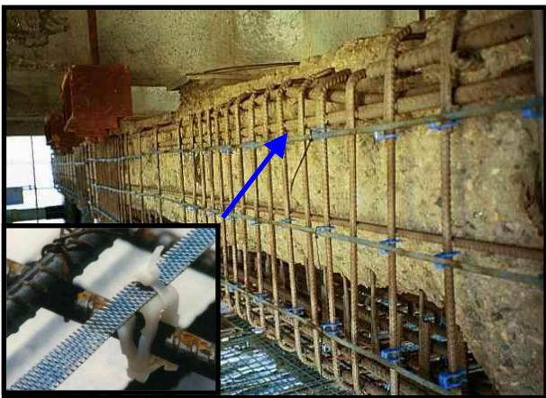
Figure 3. Ribbon mesh anodes are attached to exposed rebars on pile caps in Australia.
